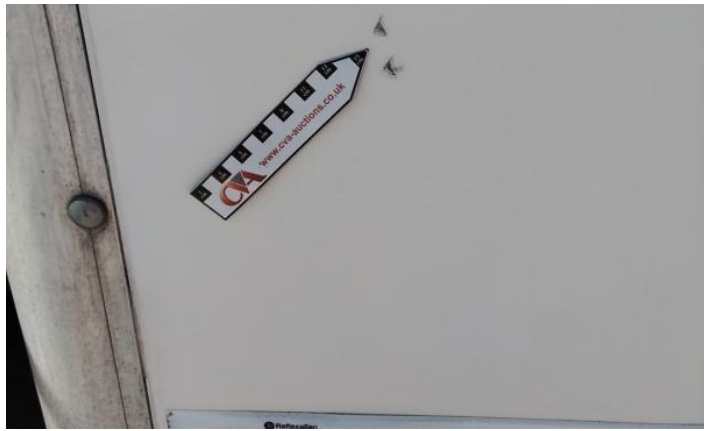
4: Door nsf Scratched Over 25mm Thru Paint
