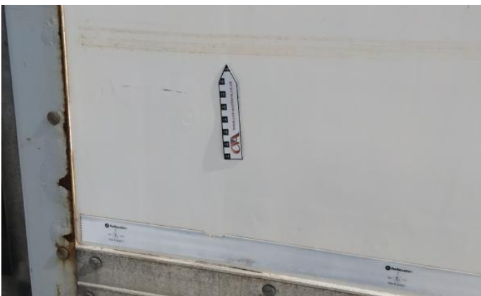
5: Door nsf Scratched Rusted
