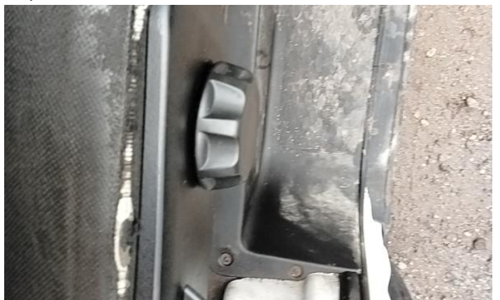
12: Switches And Controls Missing Replace
