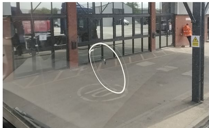
5: Door osf Dented Over 30mm
