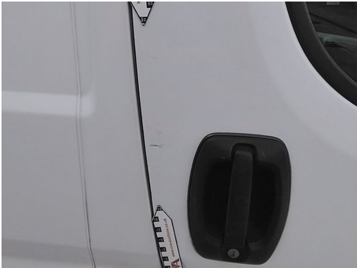
7: Door osf Scratched Over 25mm Thru Paint
