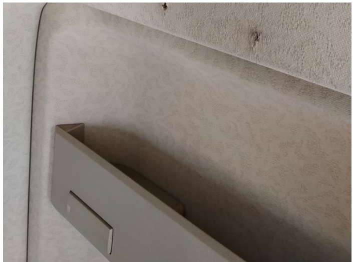
14: Roof Lining Holed Over 3mm
