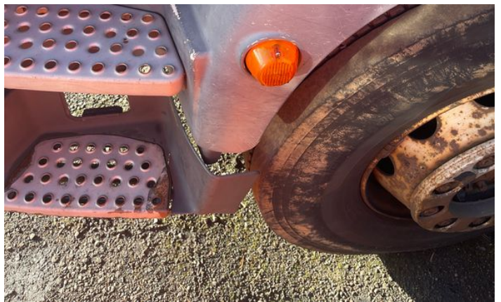
4: Wing nsf Chipped Multiple Chips
