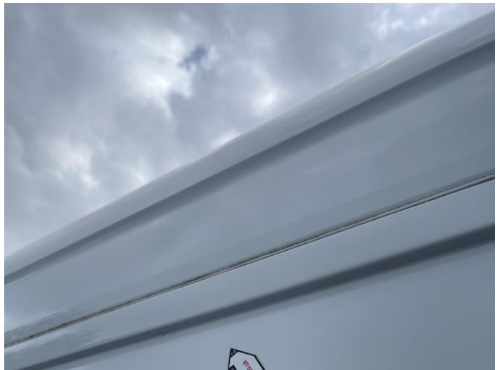
2: Roof Dented Over 30mm
