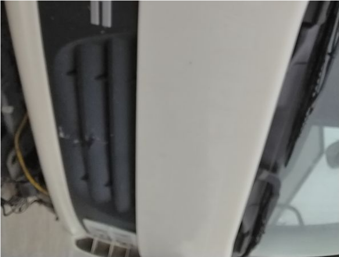
1: Bonnet Cracked Replace
