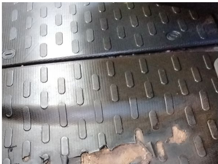
8: Carpets Front Torn Over 10mm
