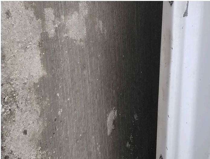
11: Sill os Dented With Paint Damage
