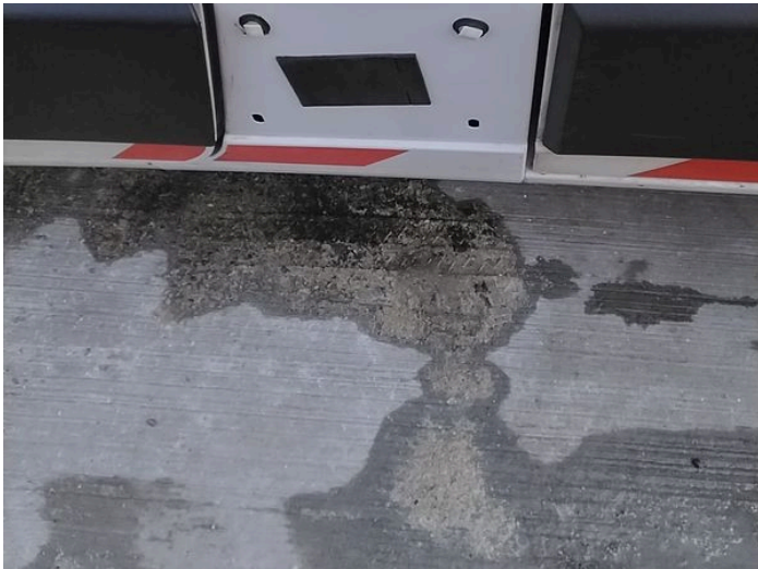
7: Door Moulding nsf Missing Replace
