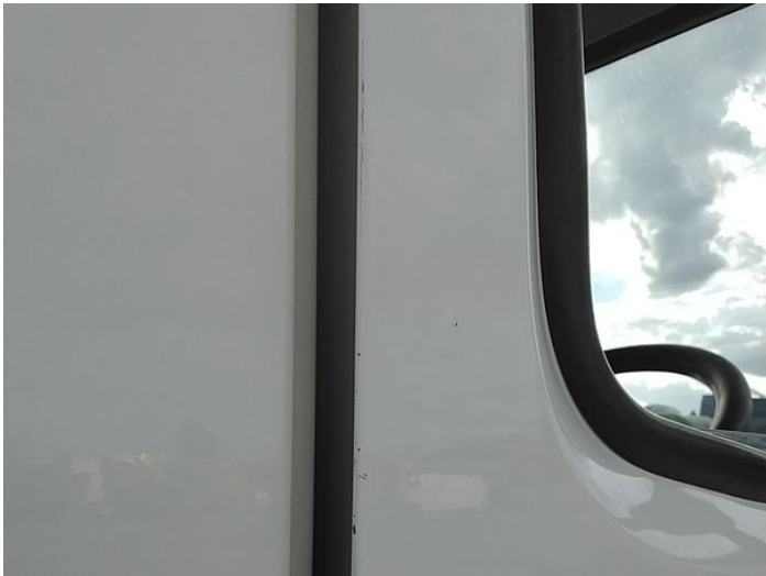
8: Door of Chipped Edge Chip
