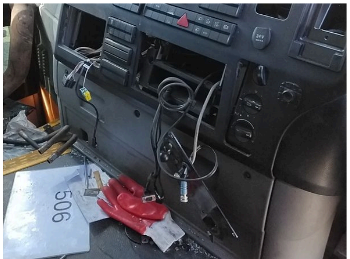
20: Switches And Controls Broken Replace
