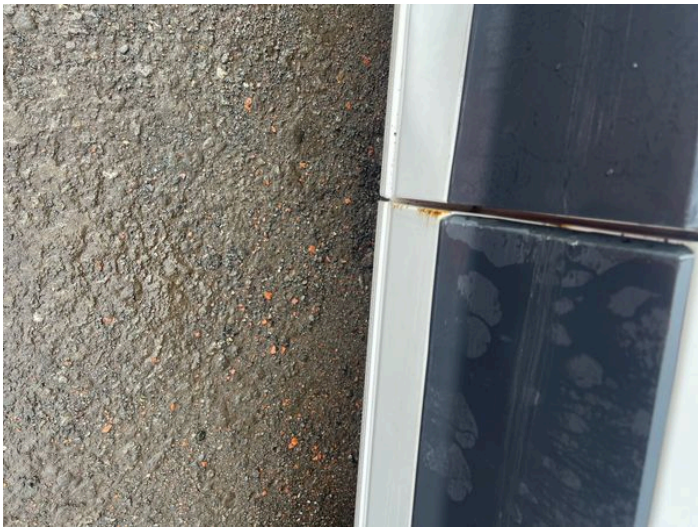
9: Sill ns Rusted Over 5mm
