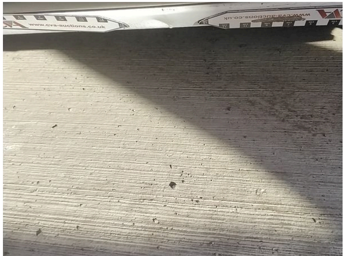
2: Sill ns Dented With Paint Damage
