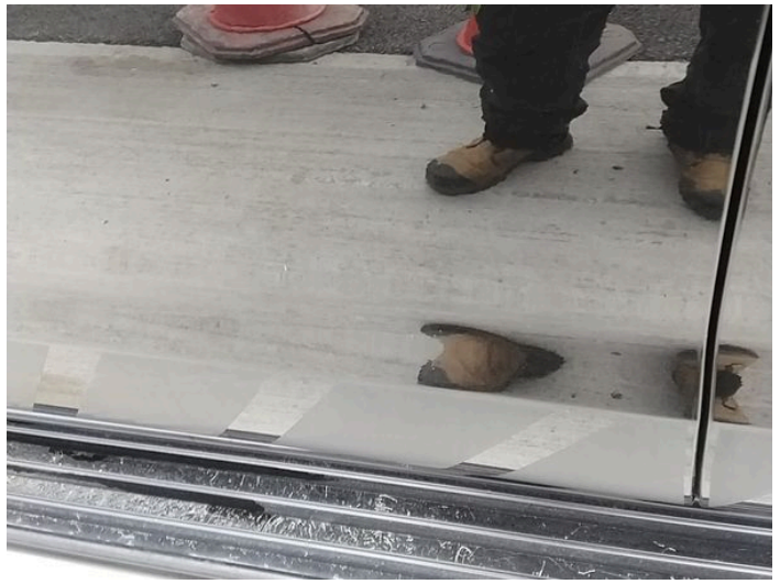
4: Door nsf Chipped Over 5mm
