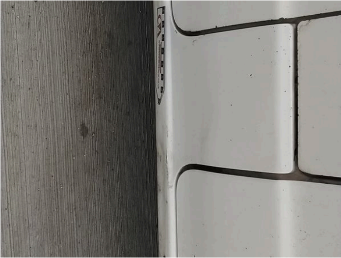
12: Sill os Dented With Paint Damage
