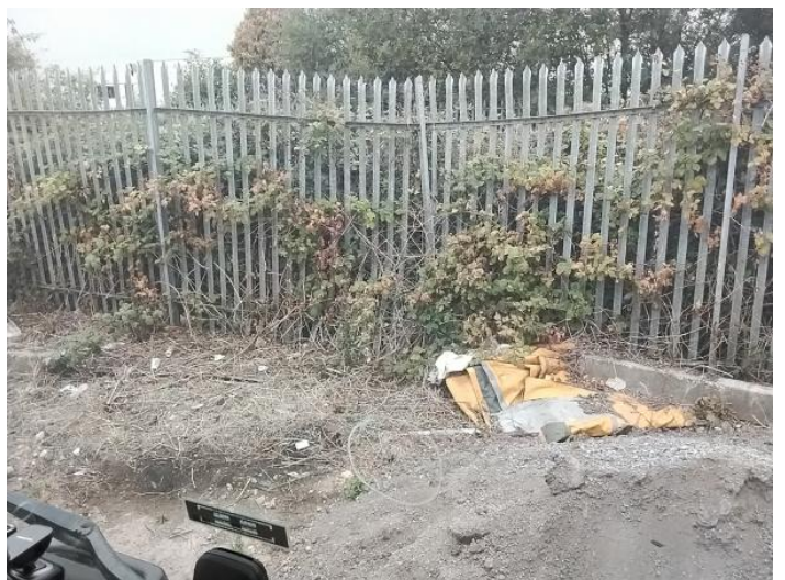
8: Screen Front Chipped Over 10mm
