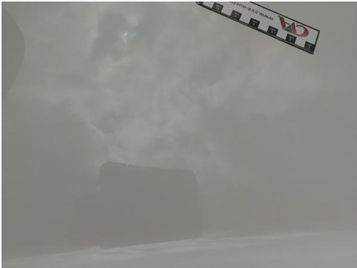
2: Door nsf Chipped 1 To 5
