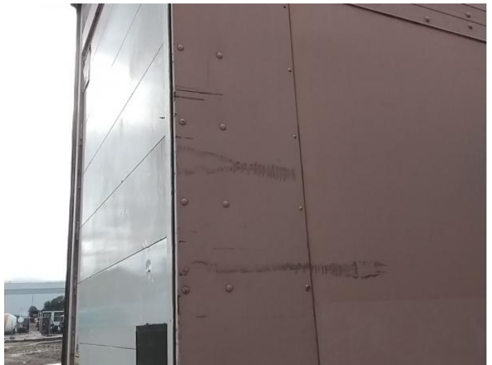
6: Qtr Panel Trim os Scuffed Over 25mm
