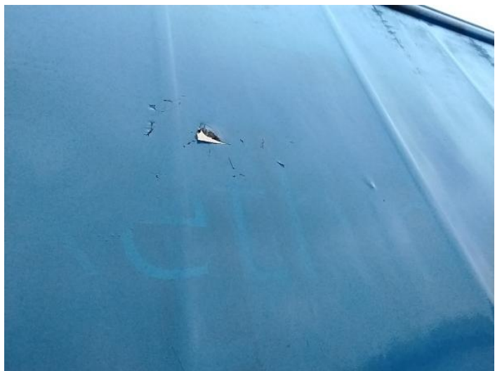
8: Qtr Panel nsr Hole Over 10mm
