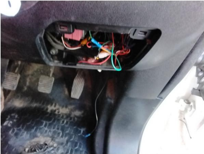
15: Fascia Panel Missing Replace
