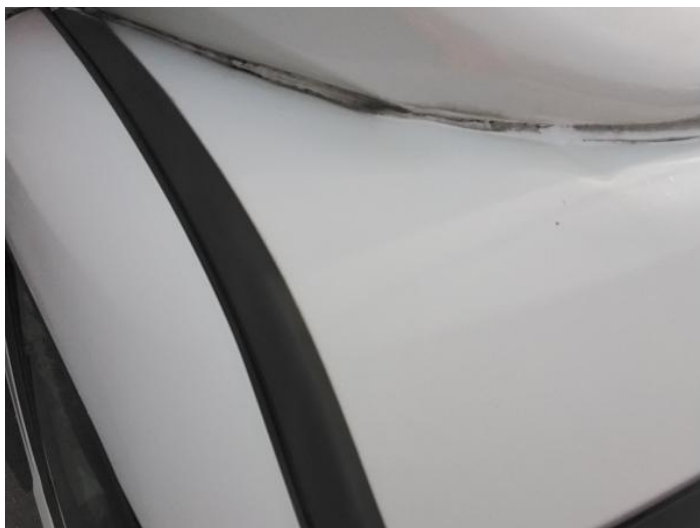
1: Roof Dented Over 30mm
